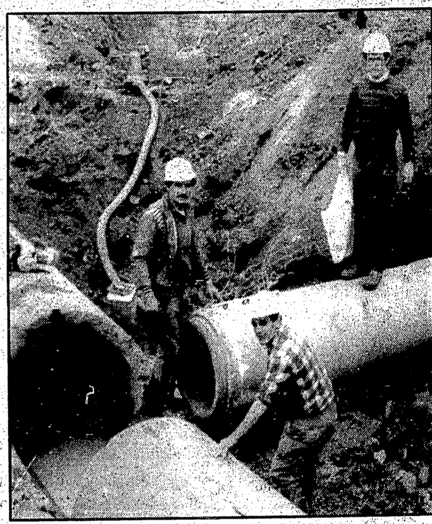
Work is underway in downtown Squamish on the sewer system. Some traffic disruption is scheduled.
