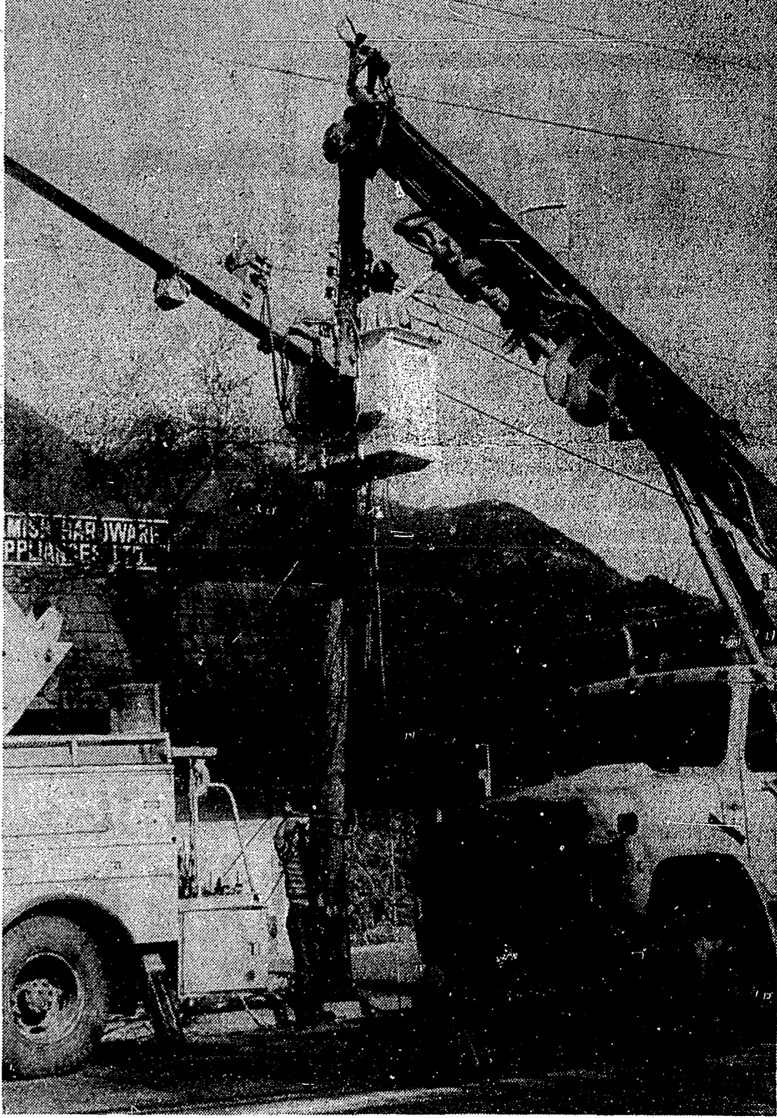
A B.C. Hydro crew arrived on the scene within the hour and quickly restored power to downtown merchants and residents.
