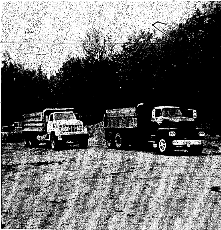
TRUCKS BRINGING ROCK to the demolition derby site during the work of preparing the area for the next derby.
