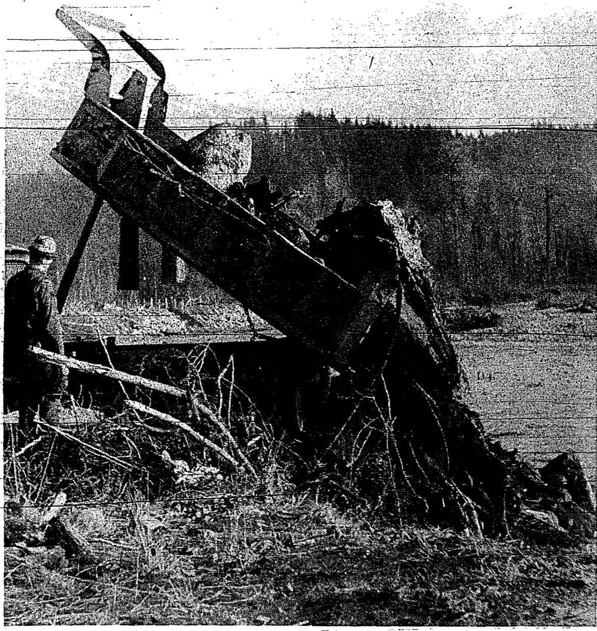
SOME of the rock and gravel which was being placed in the river east of the golf course to construct a wingdam and divert the current, is being dumped while Mike Johnson is watching. Further work will be done under a joint cost sharing plan by the district and the provincial government.
