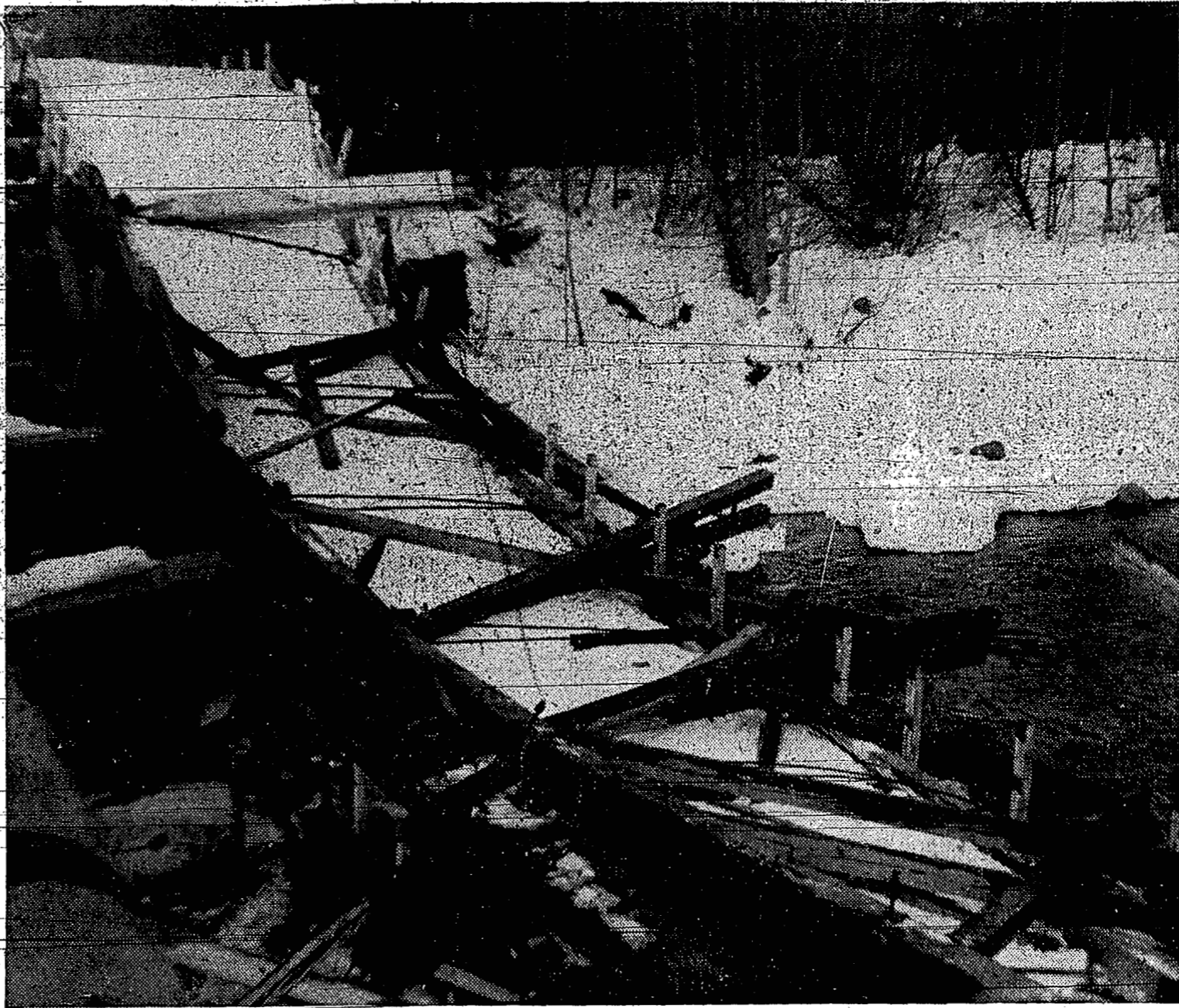
OLD CHEEKYE BRIDGE lying in the river after it collapsed last week.
