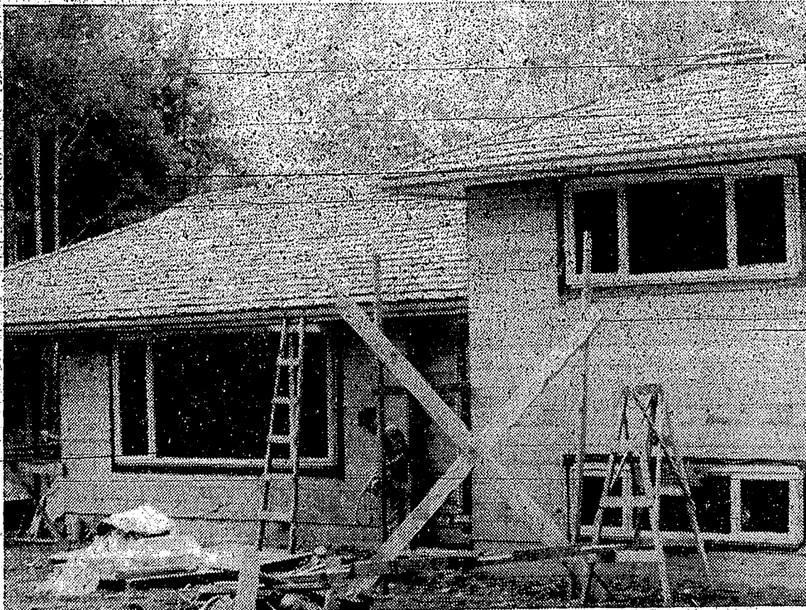
SPLIT LEVEL home in the Highlands being built for Mr. and Mrs. N. Squires by Twiss Bros. This house is located on Ayr Drive.
