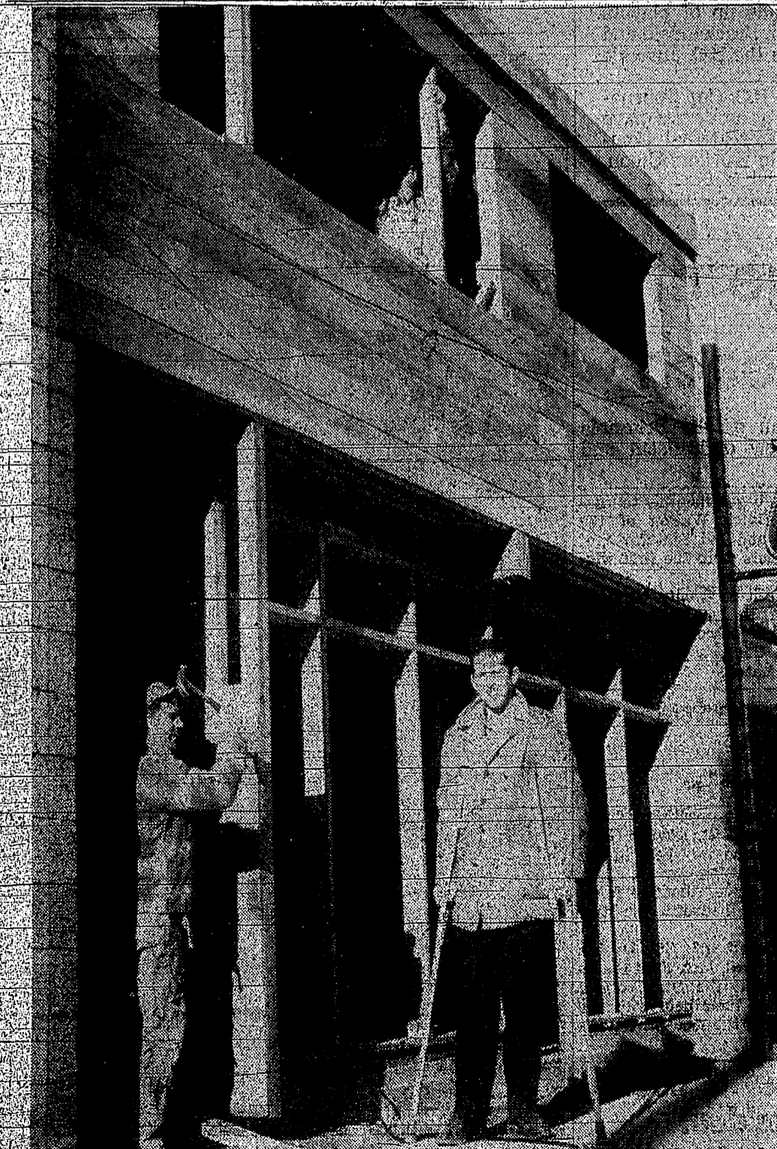
NEW STORE building of Dennis McDougall's will open in a few months under the name of McDougall's Music and Furnishings. On top floor will be two two-bedroom apartments for rent. Watching contractor Lloyd Twiss at work is the 25-year-old proprietor who started in business five years ago with the Squamish Record Shop.
