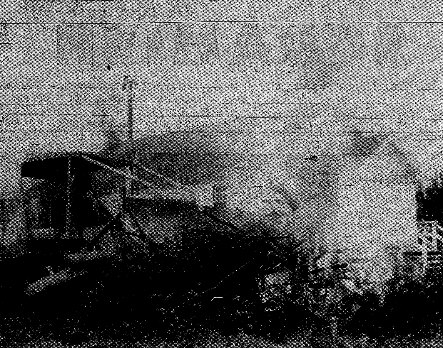
CLEARING AND BURNING for the new Christian Education Centre of Squamish United Church has now been done and tenders for construction of the
