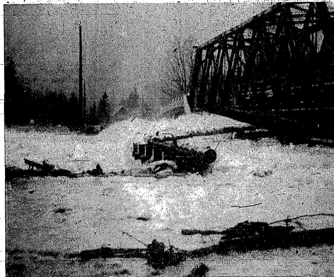
FLOODING Cheakamus River cascades over low level highway bridge at Cheekye. Old span on right has not been in use for several years since the new one, with cross timbers showing, centre, was built. Bridge withstood terrific onslaught of water and debris for 24 hours until river receded.
