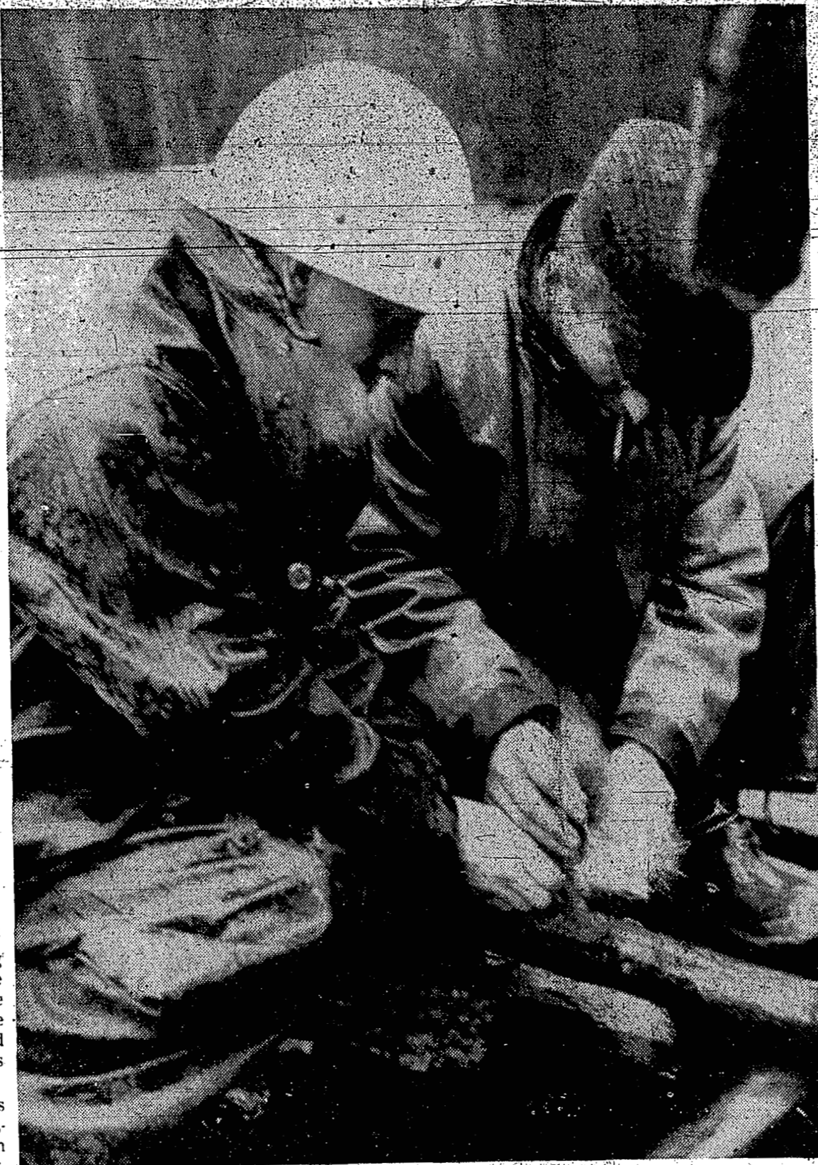
HIT BY REAL bridge-bender, at the busy trying to free the huge snag. height of the flood last Sunday the Preparing to blast the fuse is lit to 30 "PGE" Mamquam trestle keeps crews sticks of dynamite, above
